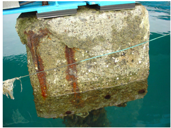
写真-3 劣化度IV
