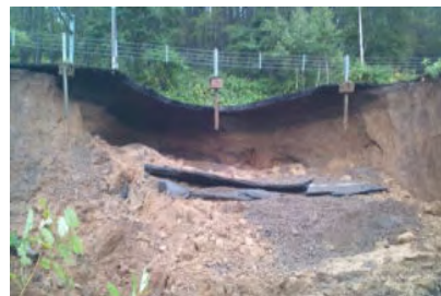
写真-2 R276伊達市大滝区法面崩壊
